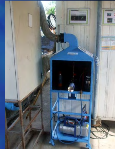
Field test for Halide torch flame test at the depot
